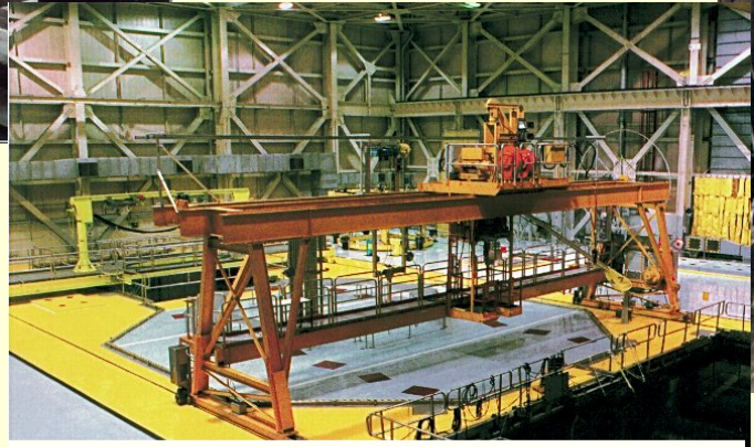
Refueling Floor & Machine
